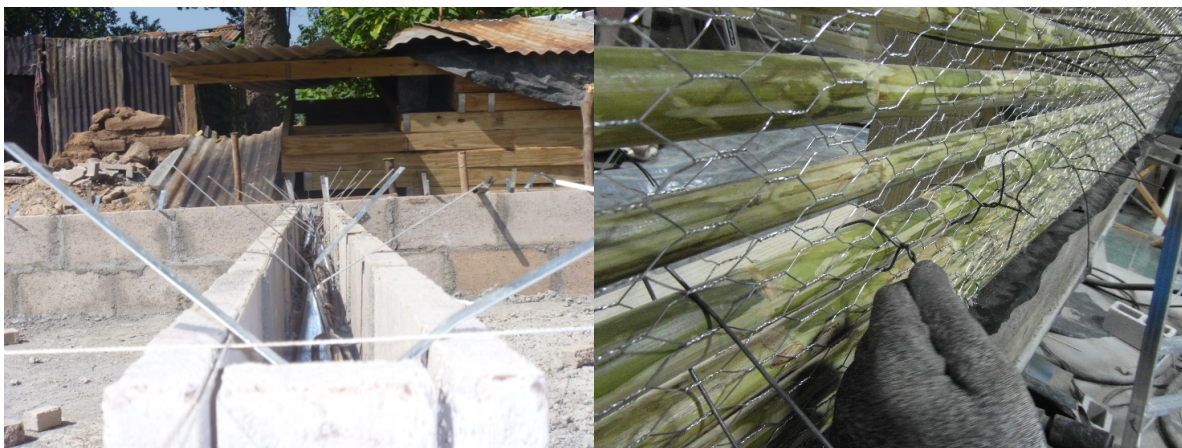
Figure 2 (L). Blockwork to timber connection detail (El Salvador Project, 2014); Figure 3 (R). Cane, mesh and wire wall detail before application of cement mortar (Kaminski, 2014)
